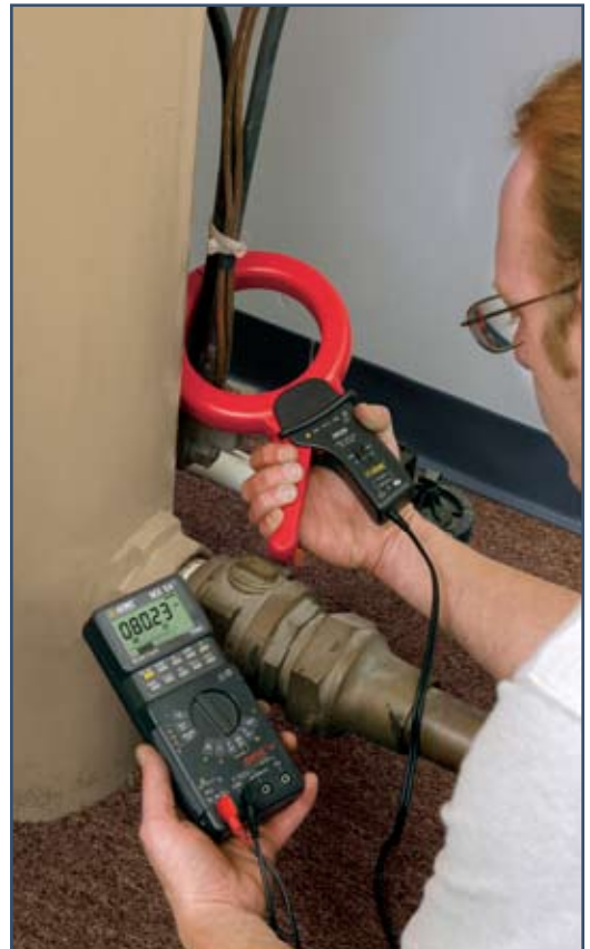
Model 2620 checking for ground fault currents
